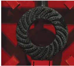
Burner Mounting screws and support bracket
